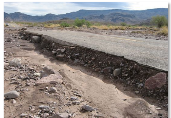
Deteriorating pavement conditions on Oatman Highway in Mohave County. Source: Arizona Central
